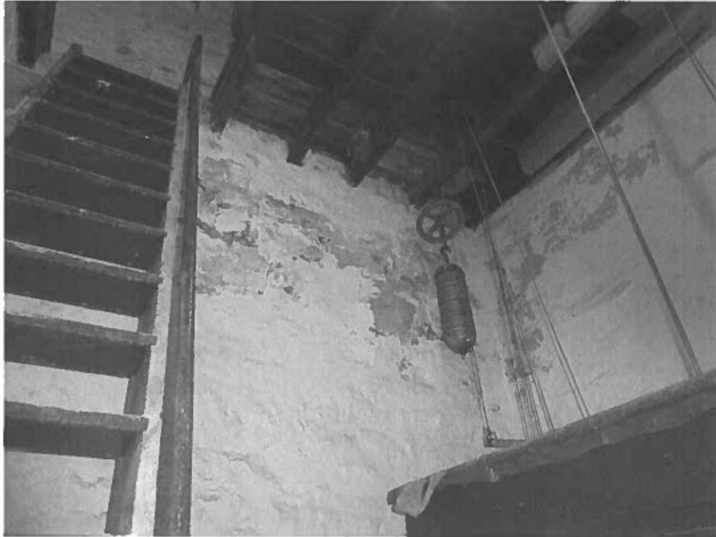
3. Peeling and flaking to west wall northwest corner.
