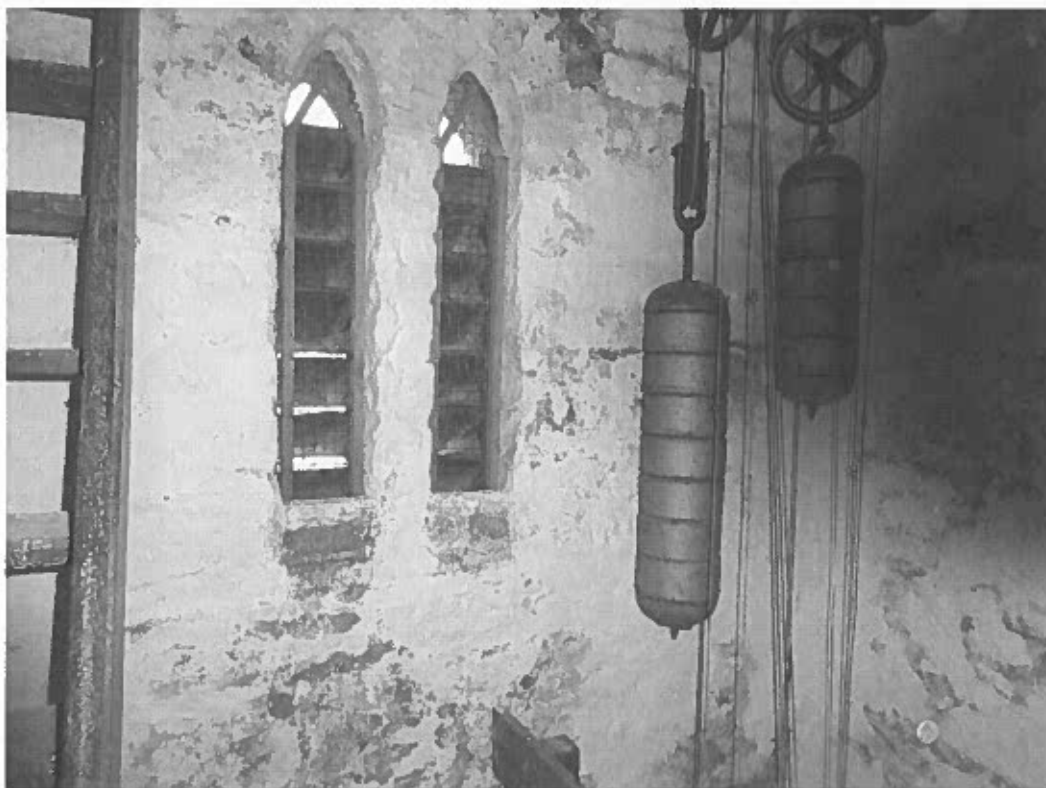
4. Discolouration and peeling due to moisture in the wall and assumed preparation issues to substrate.
