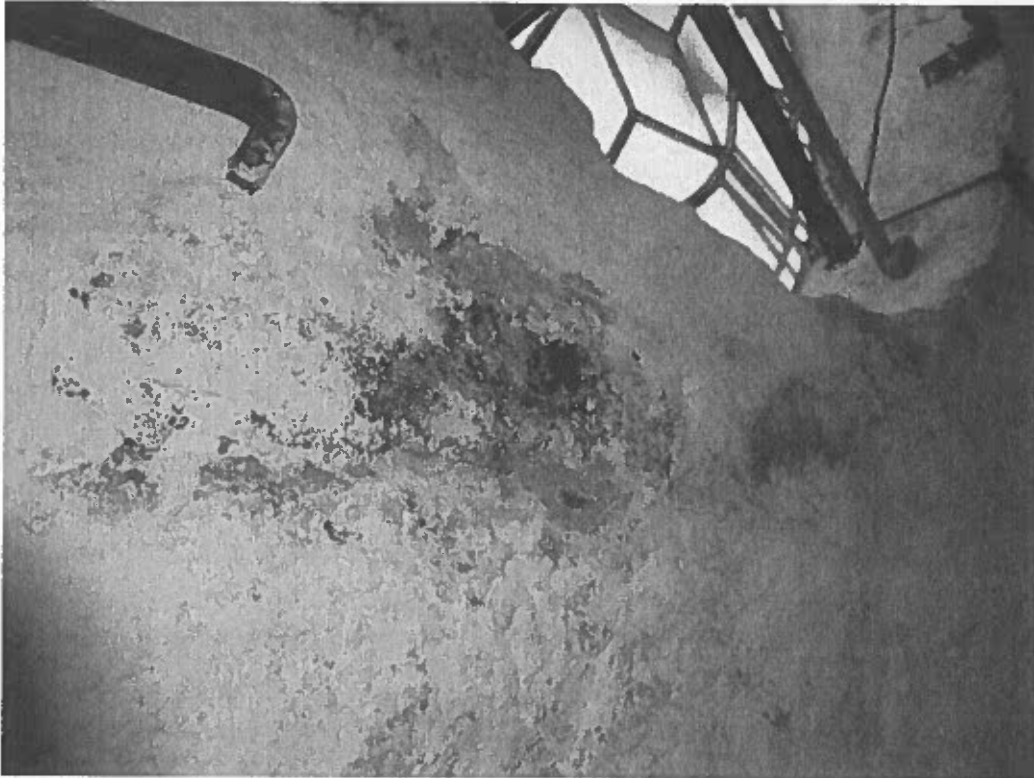
5. Evidence of cement and paint failure over certain stones.
