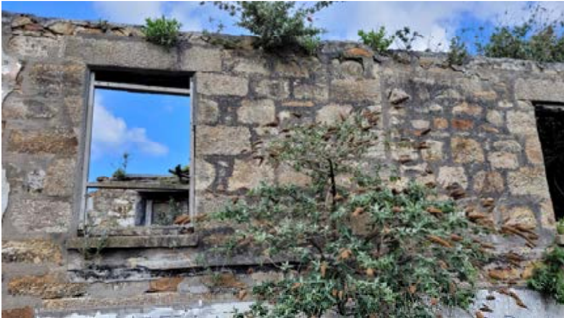
11. Vegetation growing from wall.
