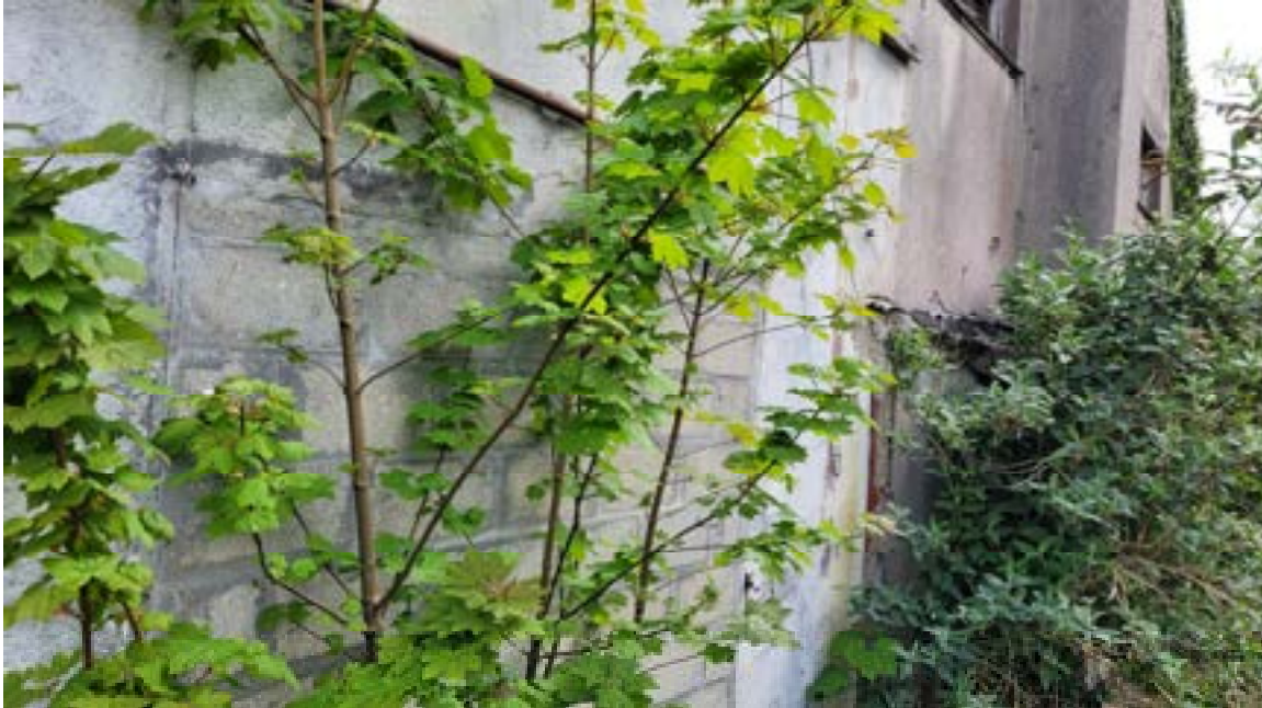
20. Opening infilled with blockwork at ground floor level on the south elevation. Note minor horizontal crack to left hand side at lintel bearing.
