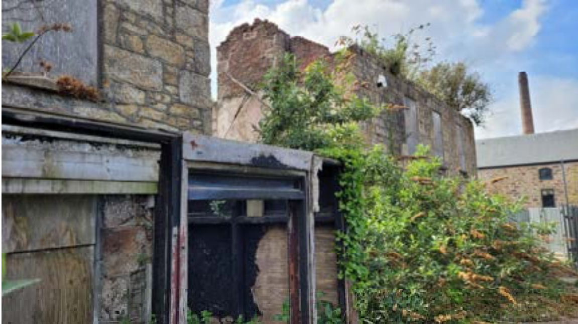
30. View on chimney showing brick panel and loose stonework to top of chimney.
