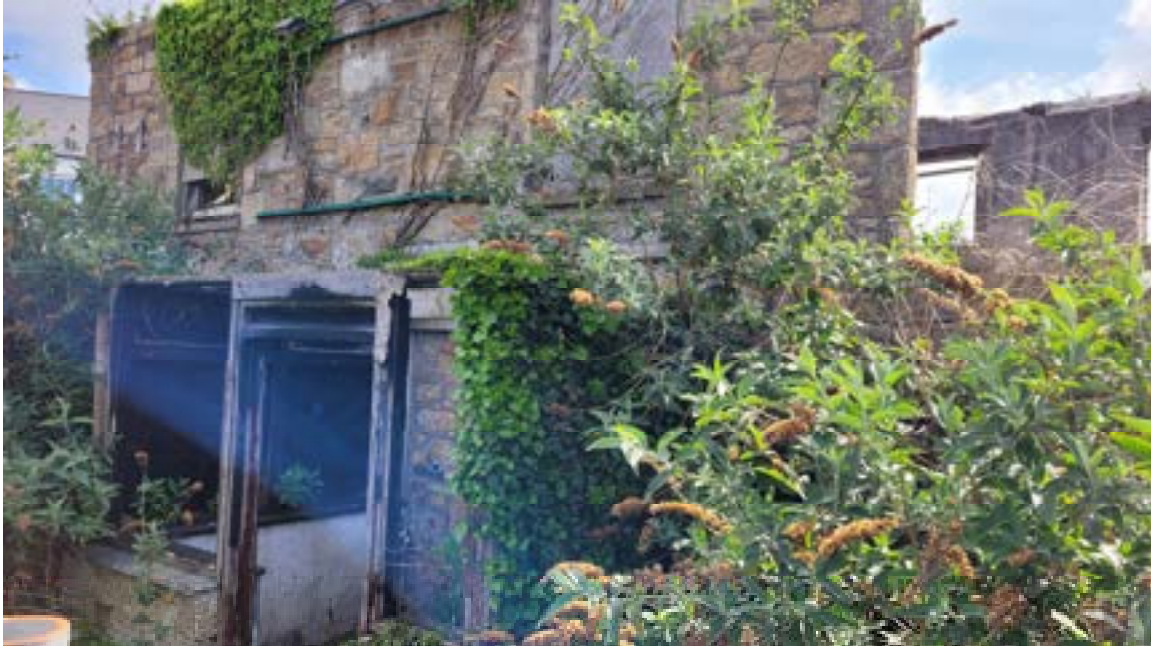
26. Fire damaged single storey lean-to with granite plinth.
