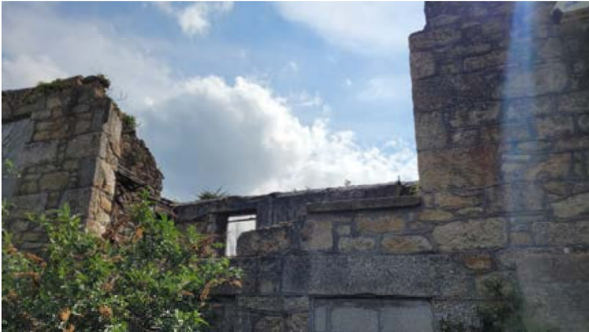
25. Collapsed section of first floor walling approximately halfway along west elevation.
