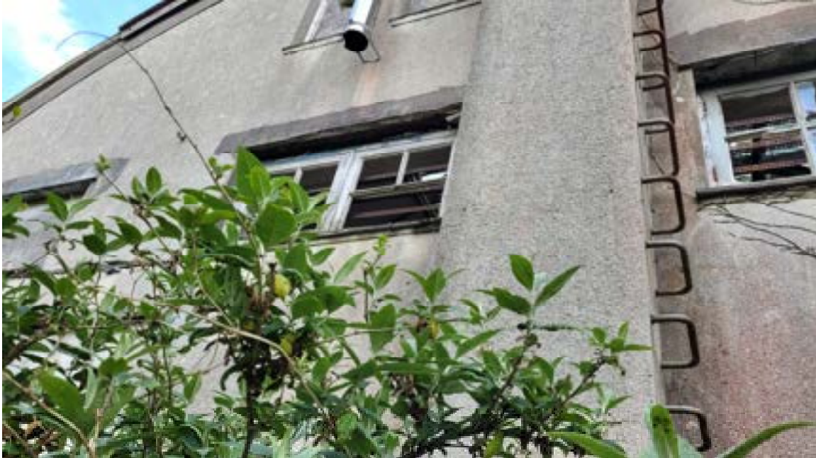
14. Corrosion to lintel soffit on middle band of window openings.
