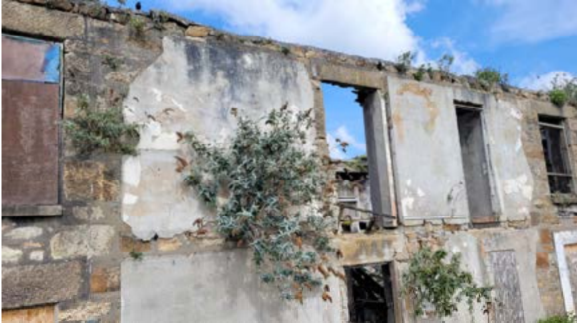
14. Crack to left hand end of first floor lintel. Walling obscured by plaster / render.
