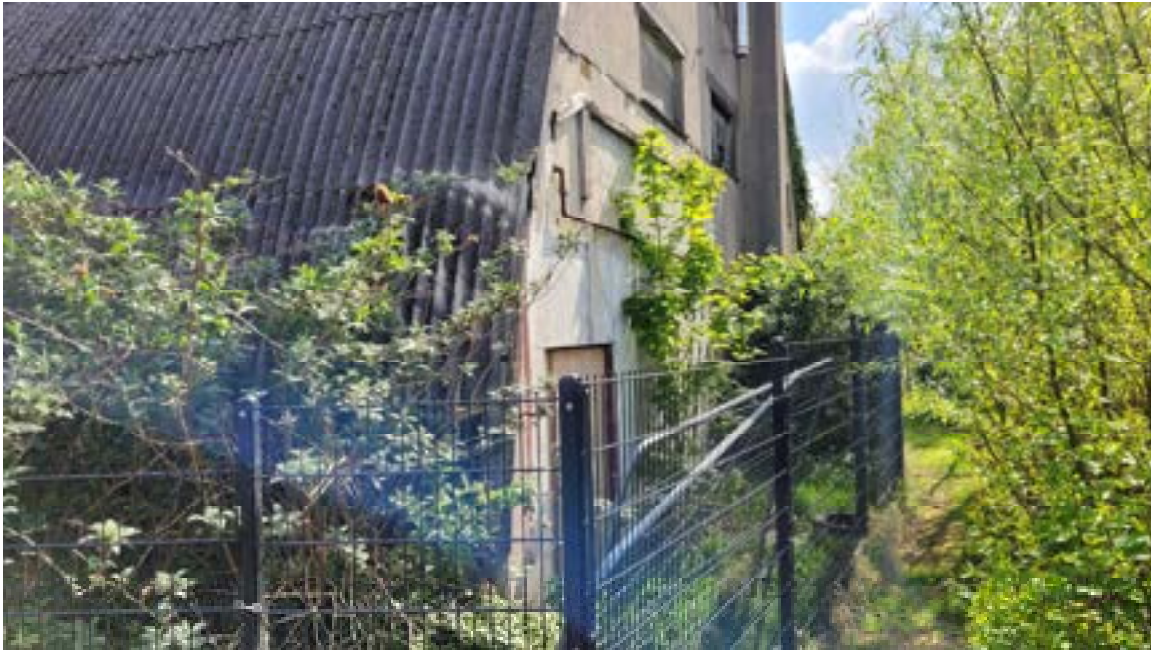
23. Damage to roof sheeting on south west corner of building.
