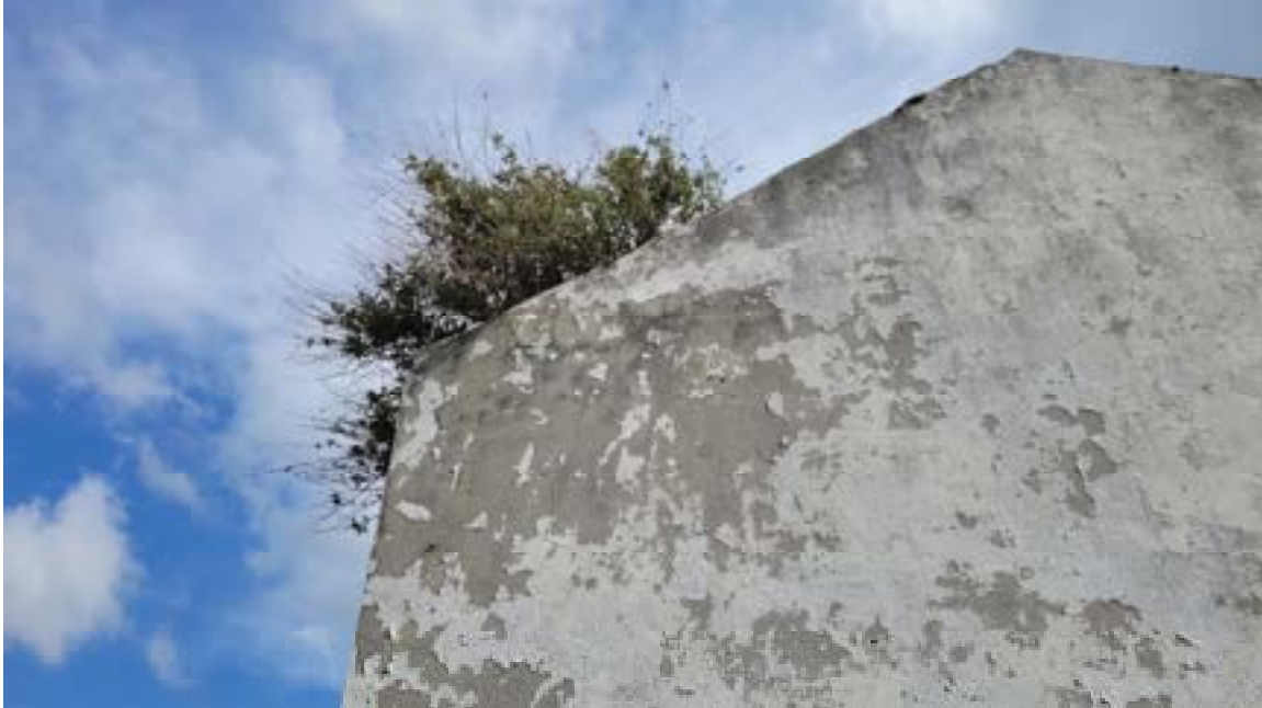
20. Cracking to top of wall adjacent to the south west corner of building.
