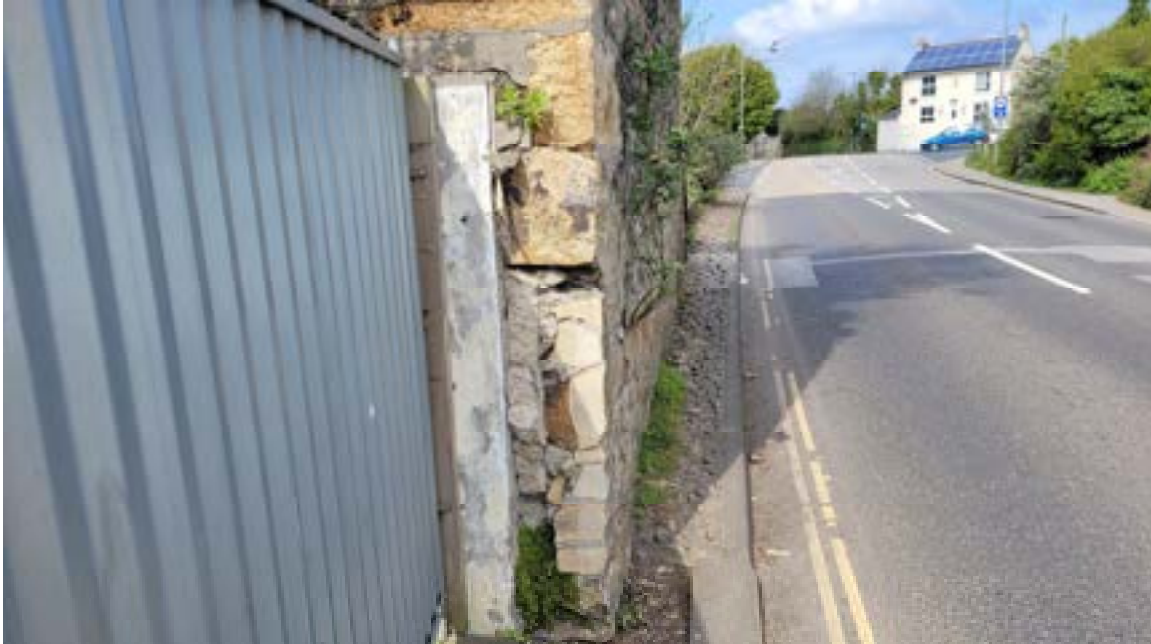
6. North east corner of building. Blockwork infill and loose stonework.
