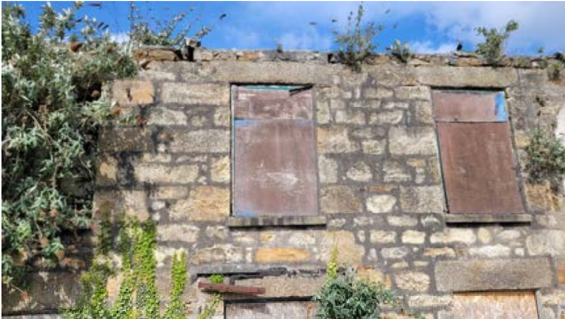
15. Loose stonework to top of wall on east elevation. Embedded metal to left hand end of ground floor lintel.
