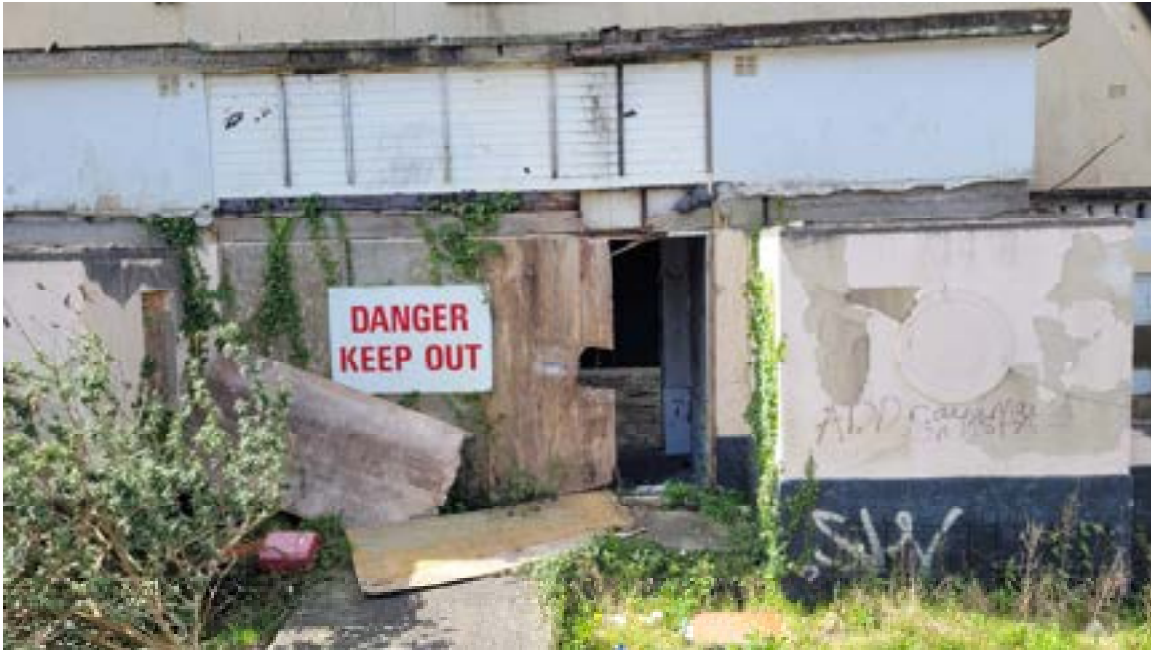
5. False timber panel above entrance with significant decay. Lintel not visible.
