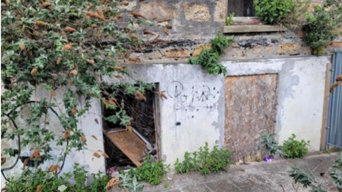
10. Vertical crack extends into render at ground floor level.
