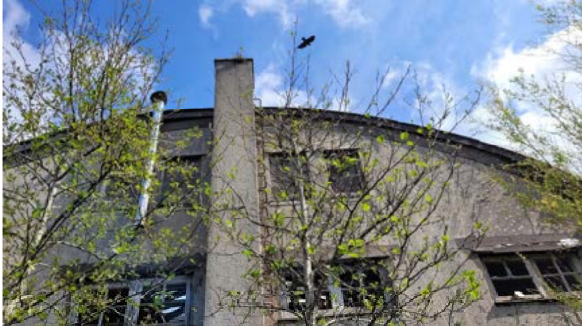
16. Vertical crack to top of chimney below vegetation.
