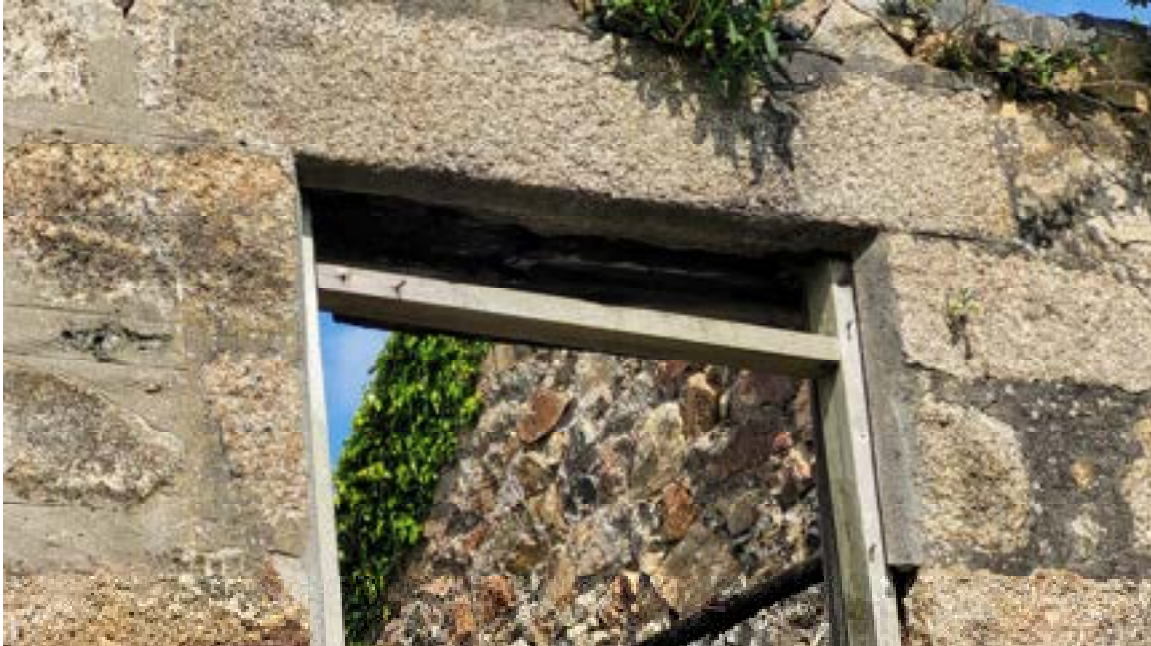
32. Close up view on lintel showing granite external lintel and charred timber internal lintel behind.
