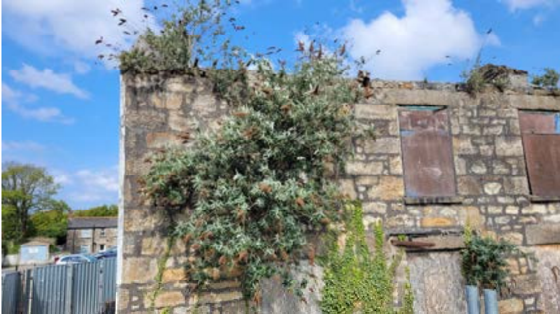
16. Vegetation obscuring window opening on east elevation.
