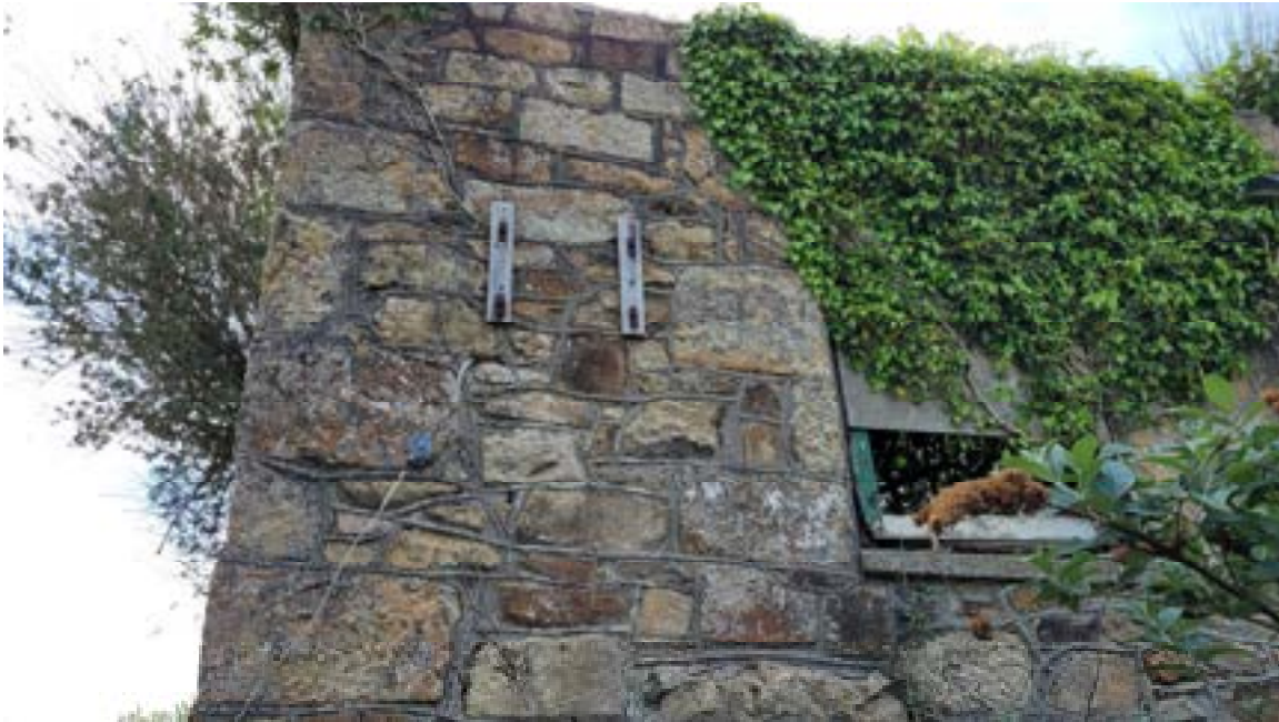
29. Timber and metal fixings secured to wall. Window opening partially obscured by vegetation to right hand side of frame.
