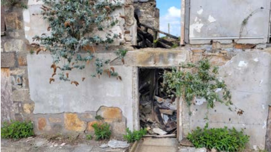
13. View into inside of building showing charred rubble.
