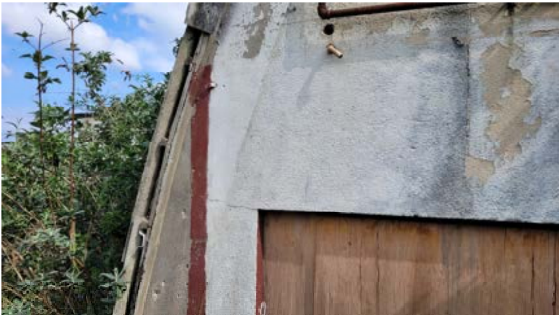
22. Minor horizontal crack propagating from ground floor opening adjacent lintel to south west corner of building on south elevation.
