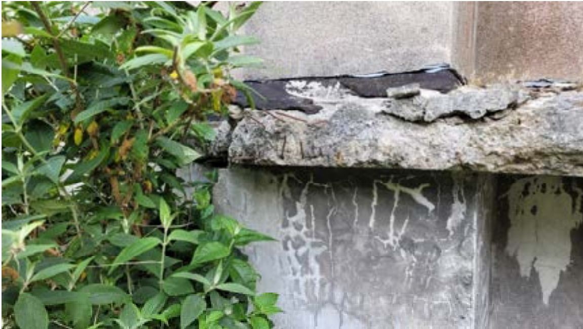
19. Degradation of concrete slab adjacent to chimney.
