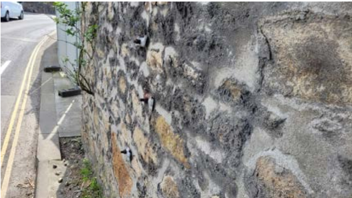
4. Fixings embedded in the north elevation potentially from previous scaffold installation but checks required to ensure these are not securing the stonework.
