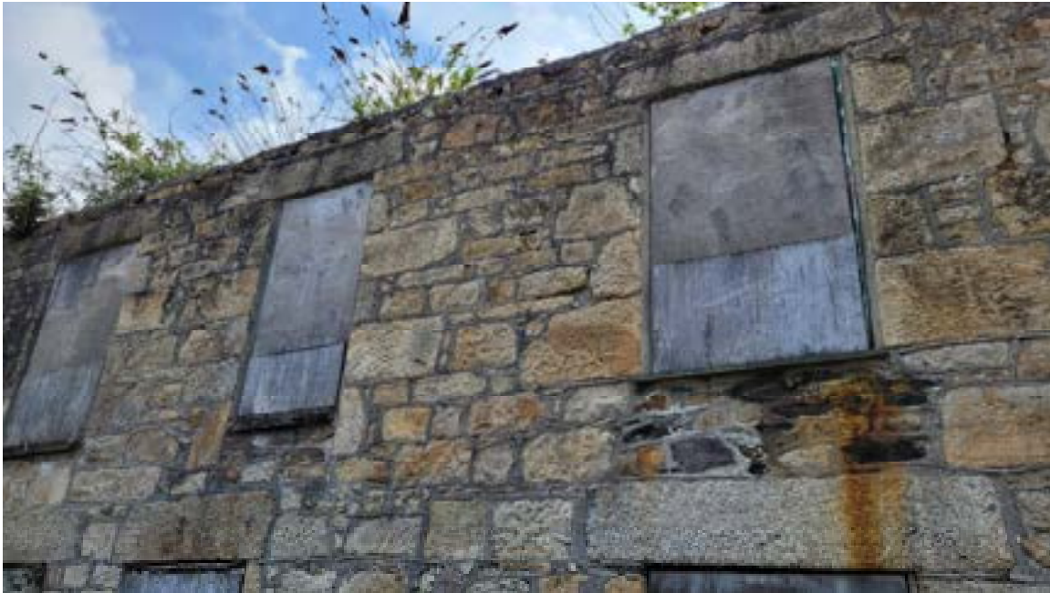
23. Cracking to left hand end of lintel over ground floor doorway and staining on stonework between the first floor and ground floor openings.
