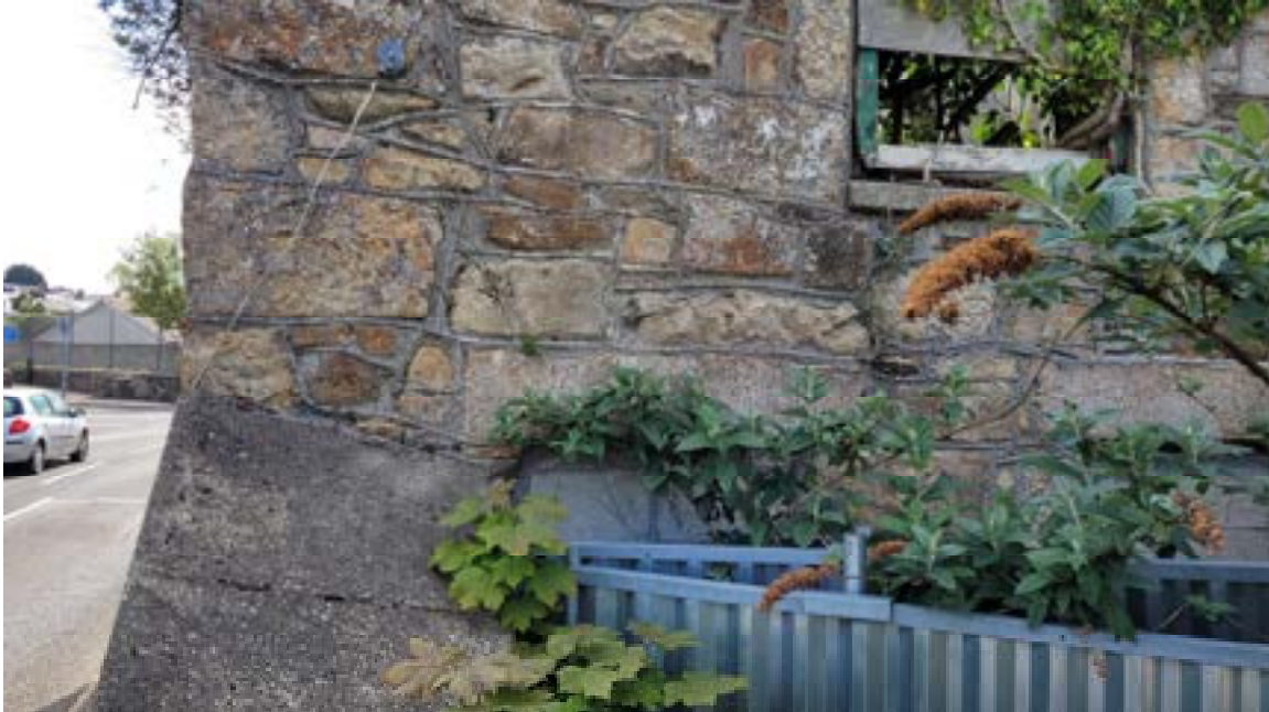
28. Minor cracking in mortar below cill. Ground floor window opening blocked up towards bottom of frame.
