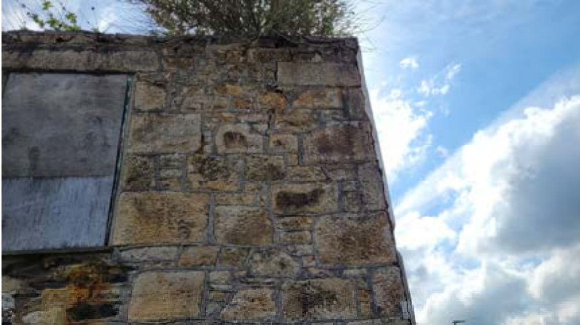
22. Cracking on west elevation adjacent to the south west corner. Note gapping between render on south elevation and wall.
