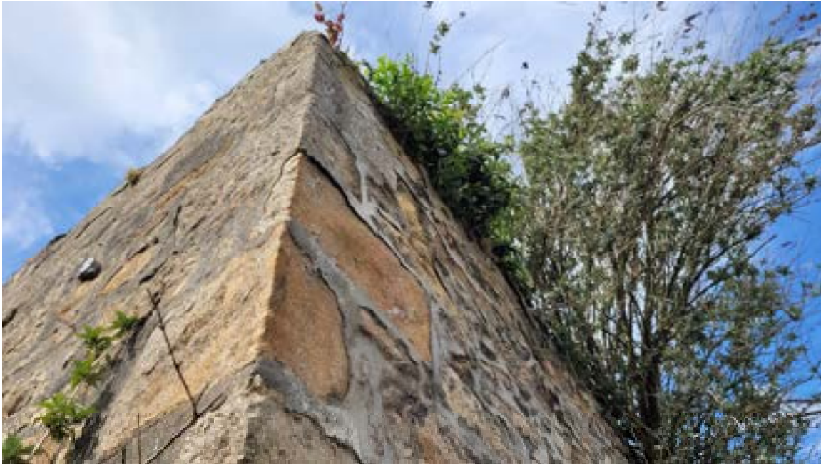
5. Gapping between mortar and stonework on north elevation.
