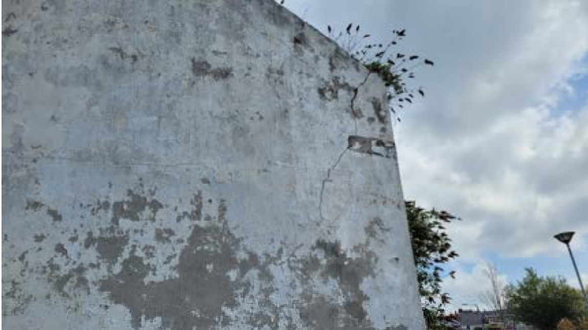
18. Cracking on south elevation adjacent to south east corner.
