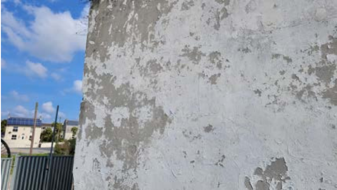
19. Minor crazing to render. Investigation required to determine whether this extends into the stonework beyond.
