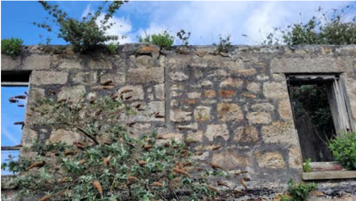
9. Vertical crack and loose stonework to top of wall.
