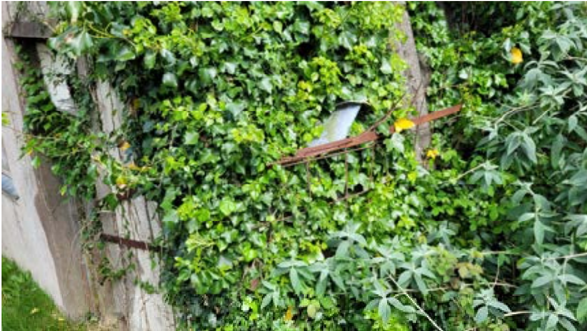
11. Metal strapping secured to wall on south east corner of building.
