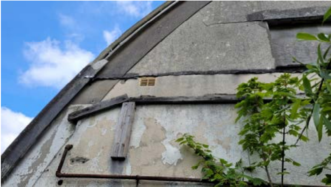
21. Degradation of roof sheeting on verge. Horizontal crack propagating from lintel bearing becoming vertical. Timber and metal pipework fixed to wall. Note chase in wall above these.
