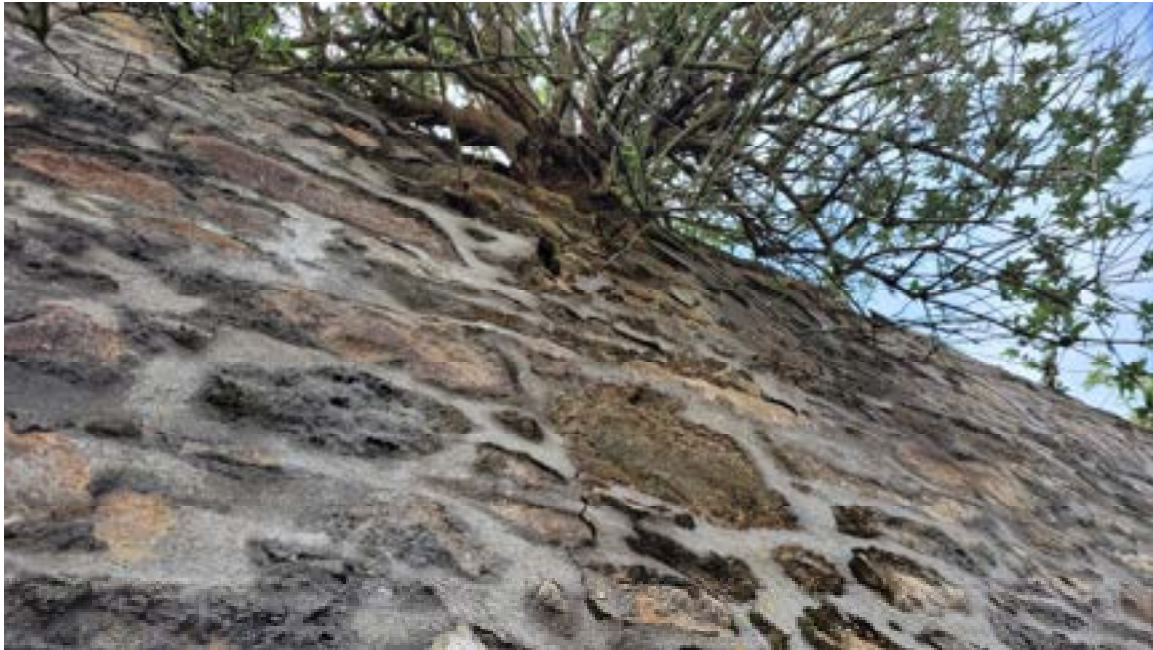
3. Damage to stonework on north elevation.
