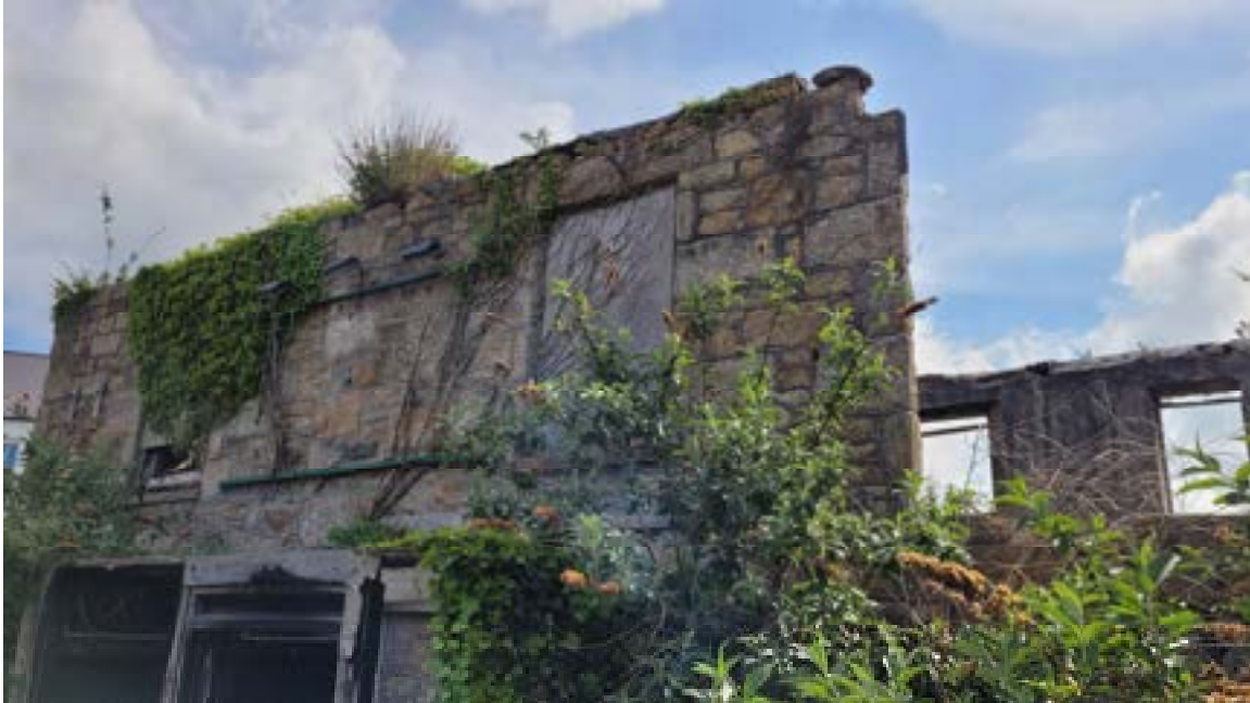
27. Loose stonework at top of the wall and metal angles fixed to the wall. Potential failure and past repair to granite lintel.
