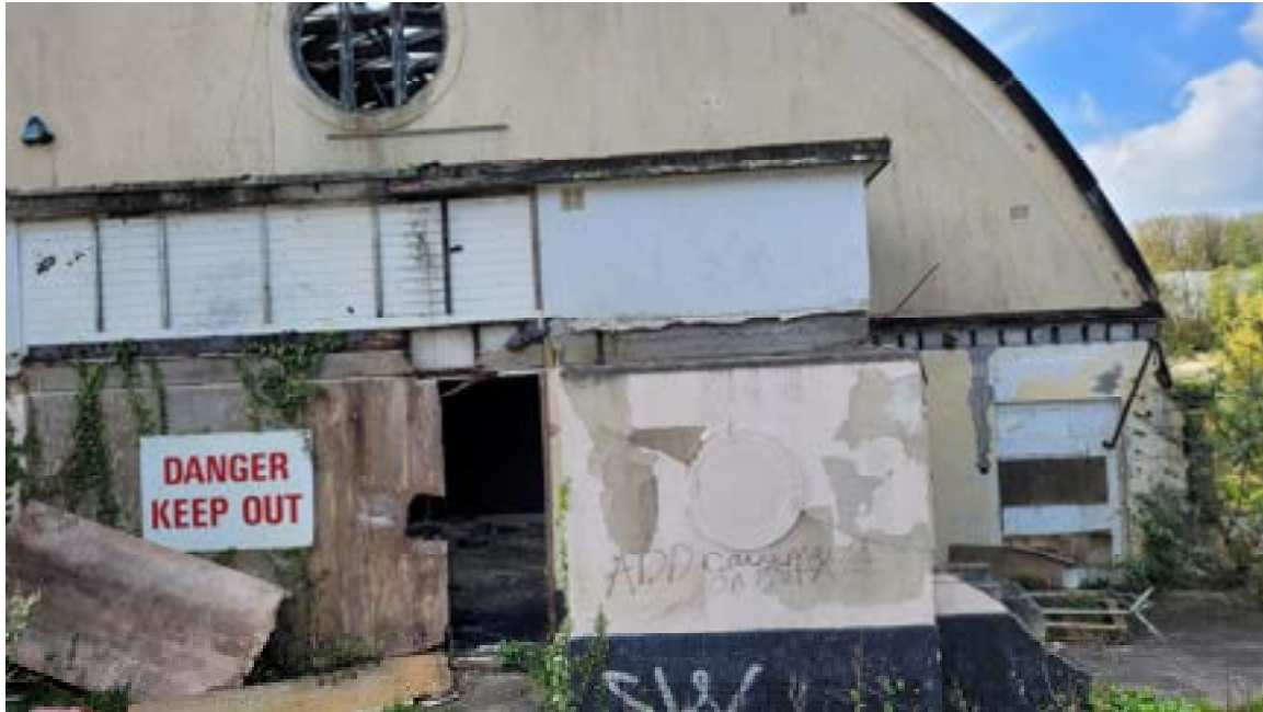
3. Pockets in wall where joists in wall appear to have been previously built in.
