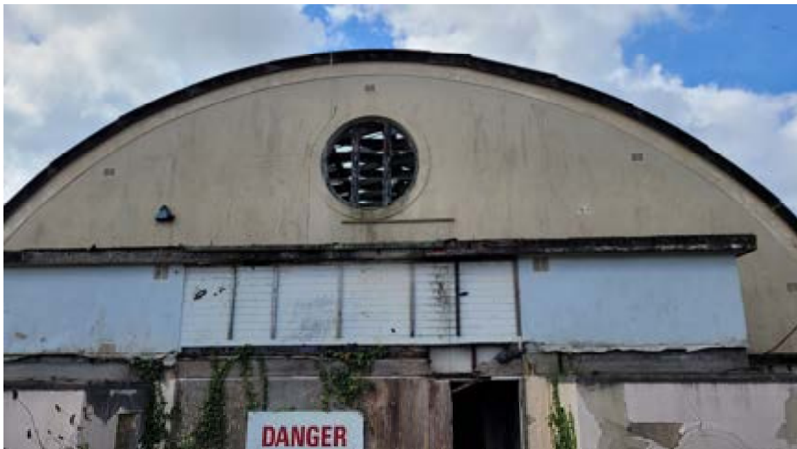
4. View on circular window opening showing vertical crack below. Note concrete roof slab below.
