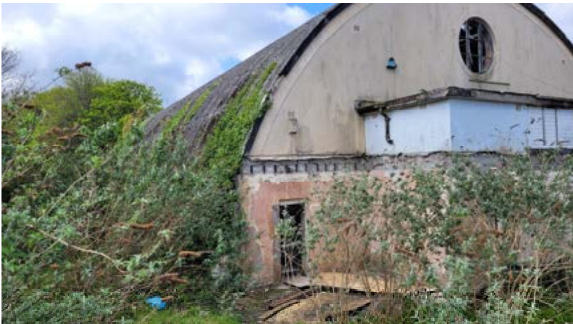
6. Evidence of joists previously built into wall and diagonal becoming vertical crack to left hand side of flat roof slab.
