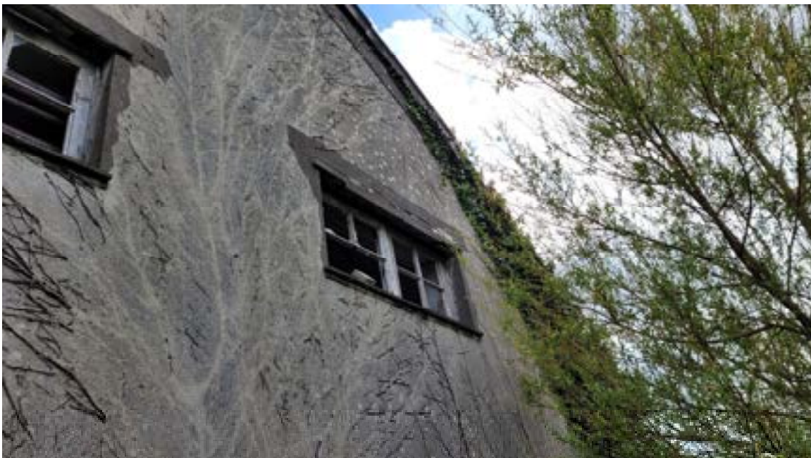
12. Failed lintel due to corrosion.
